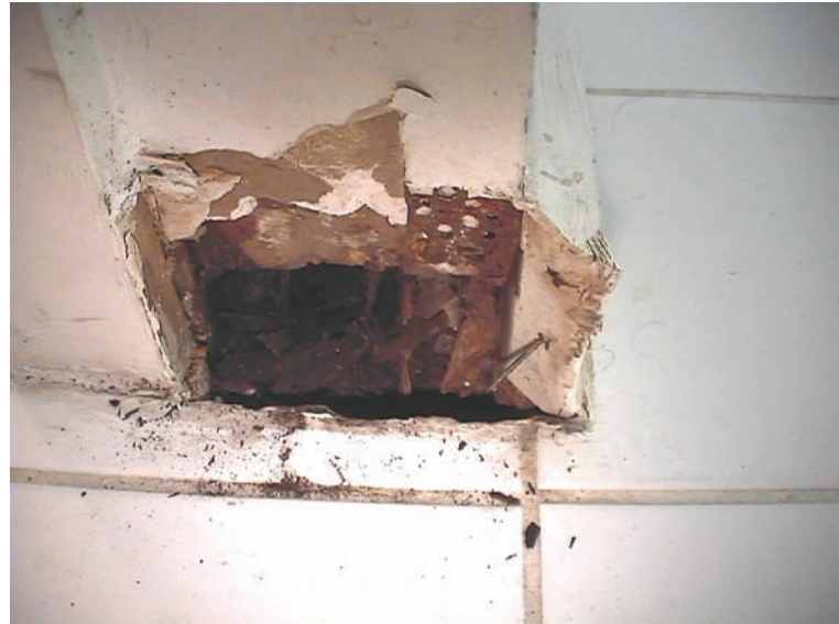
Figure 1 Water damage to bottom plate of separating wall
