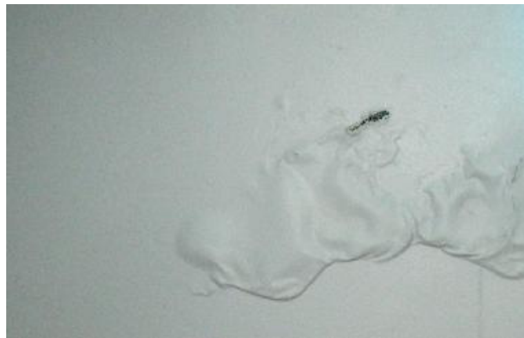
Figure 4 – Internal damage to a wall from water vapour transmission
