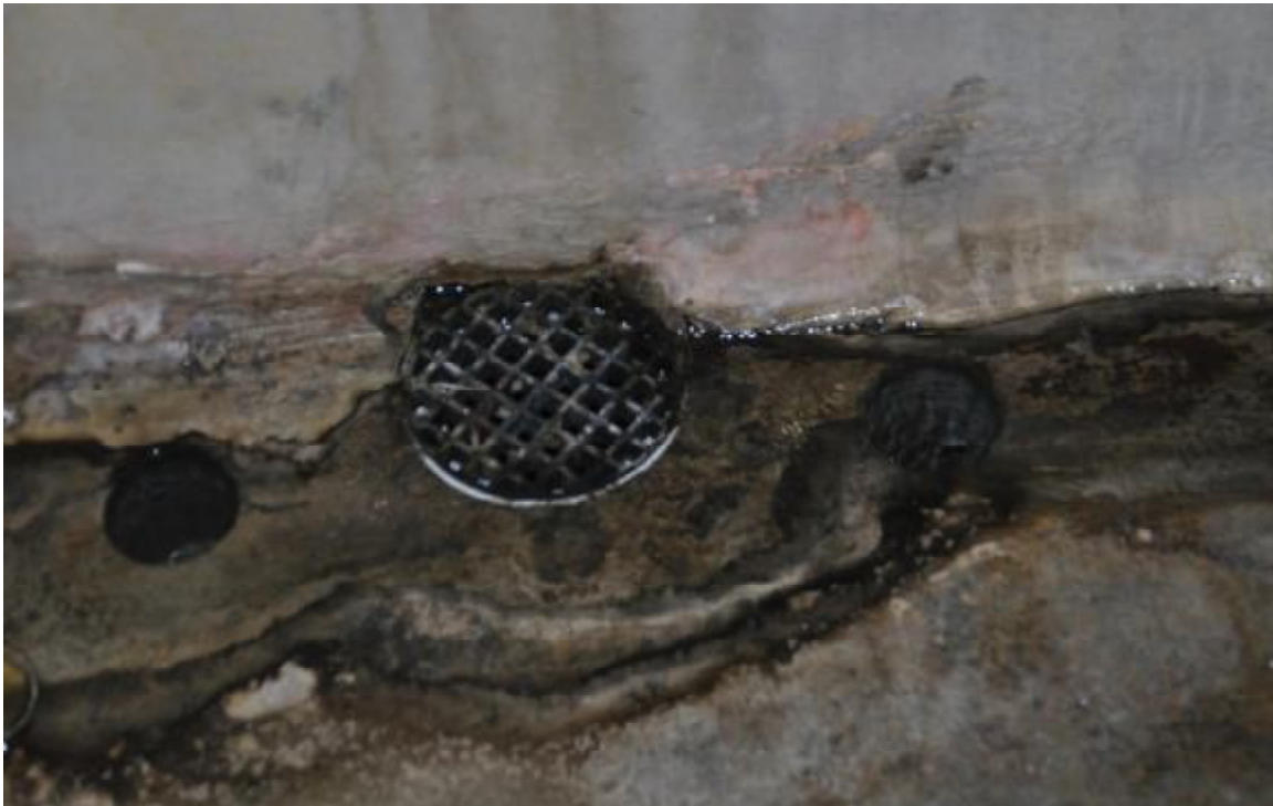
Figure 1 – Drainage along wall of underground car park
