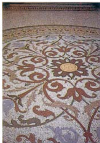
Ornate mosaic floor of the Block Arcade, Melbourne showing wide gaps between irregular shaped tiles.
