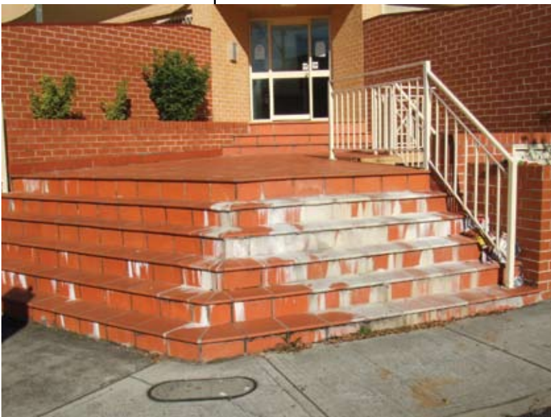
Photo 1. Secondary efflorescence with calcium carbonate forming on the surface of external stair tiling.
