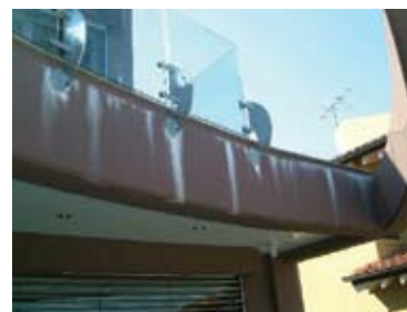
Photo 6. Where the gradient in the substrate leads to a free edge, efflorescence will form on the riser. To avoid this problem, seal a water-stop angle to the floor at the edge or one tile in from the edge, and grade the substrate behind the angle to a drain.
