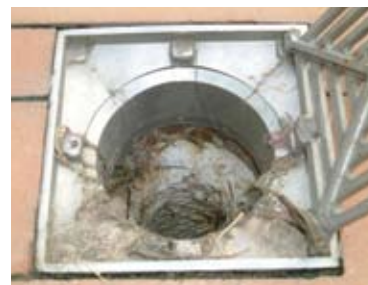
Photo 5. When the drain is open at the neck, and there is a gradient in the substrate to the drain, the efflorescence forms down the drain pipe and not on the tiles.
