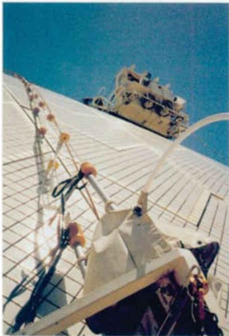
A close-up of the remedial works which include replacement of 17 kilometers of sealant
