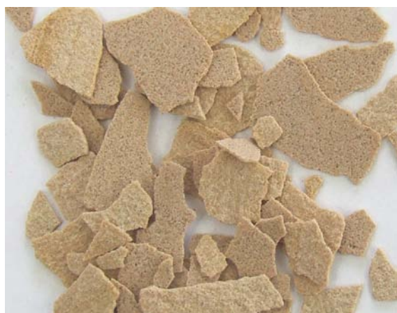
Flakes of sandstone that have spalled from sandstone paving which had been treated with an impregnating sealer. The flakes retained their water repellency while the underlying stone was unaffected.
