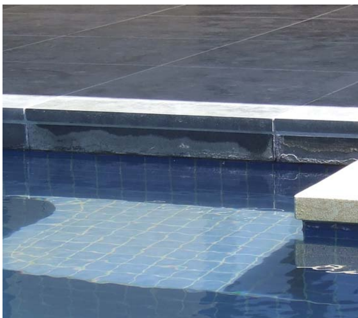
Delamination decay of sealed stone used as a pool edging. Although this stone had been tested and found to have a very high resistance to salt attack, the use of a sealer has affected the dimensional stability of the stone's surface in wetting / drying situations.
