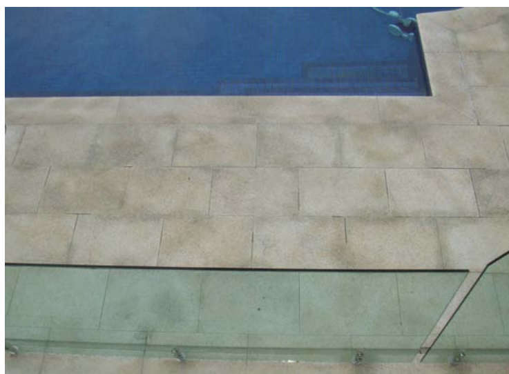
Efflorescence has formed inside this granitic stone and it is now irremovable. Pre-sealing the back of the stone with a specialist solution could have avoided this problem.
