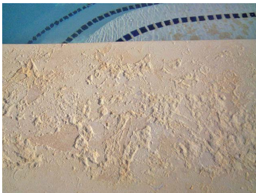
Salt spalling on travertine around a salt water pool after only 5 months
